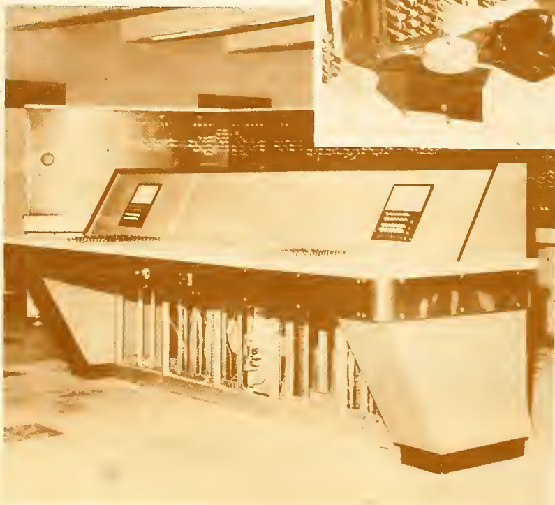
Painéis de Controle — CTC — EFSJ
